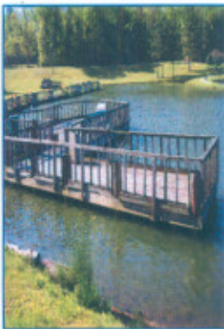
RWSIR's #1 Priority for 2011 is the Camp Dream Dock Project—plans are moving forward to begin demolition & renovation!
